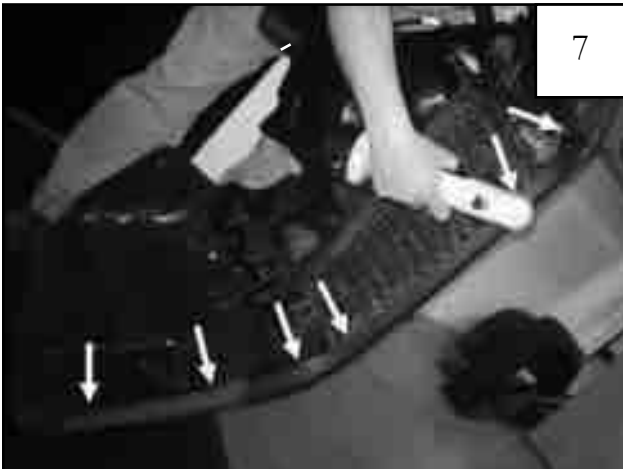
Use a drill with a 5/16" bit to drill through six plastic rivets along edge of flare/splash shield. Discard the flare, but retain the splash shield and inner structure with light attached.
